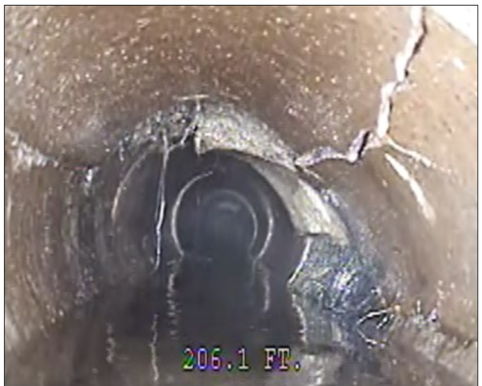
Many pipes in the Rocky Ford wastewater system are subject to infiltration and in need of replacement.
