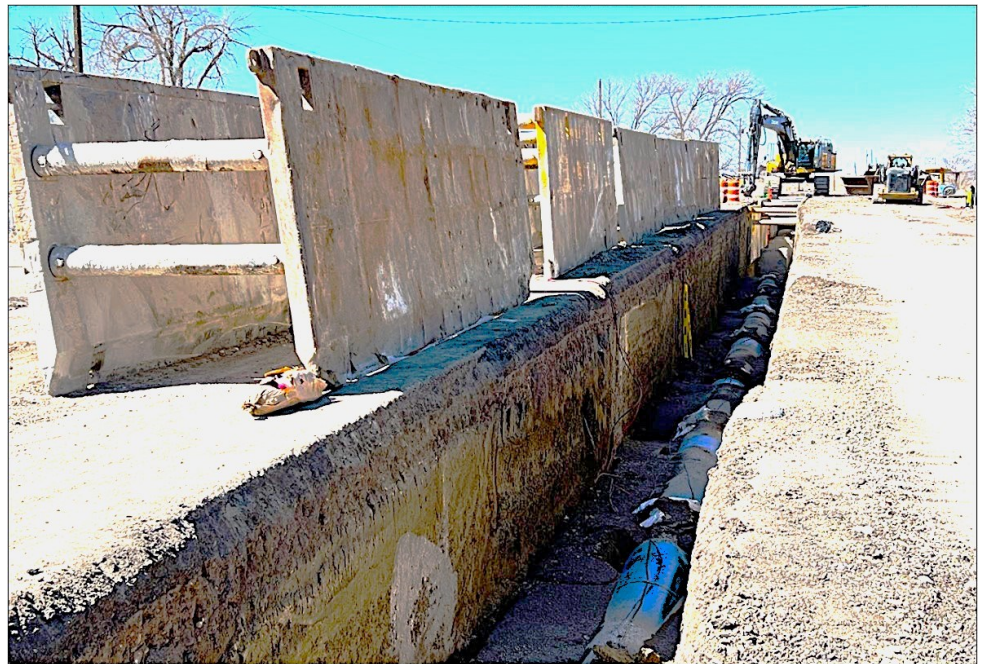
Pate Construction is installing the AVC pipeline on State Highway 96 at the west side of Boone.
