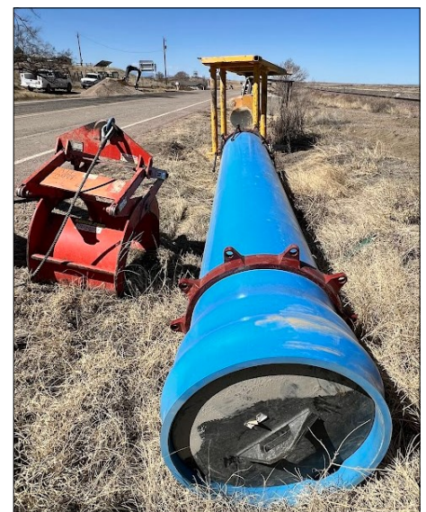
The PVC pipe under State Highway 96 is mechanically restrained with a steel collar and bolts at the joints.
