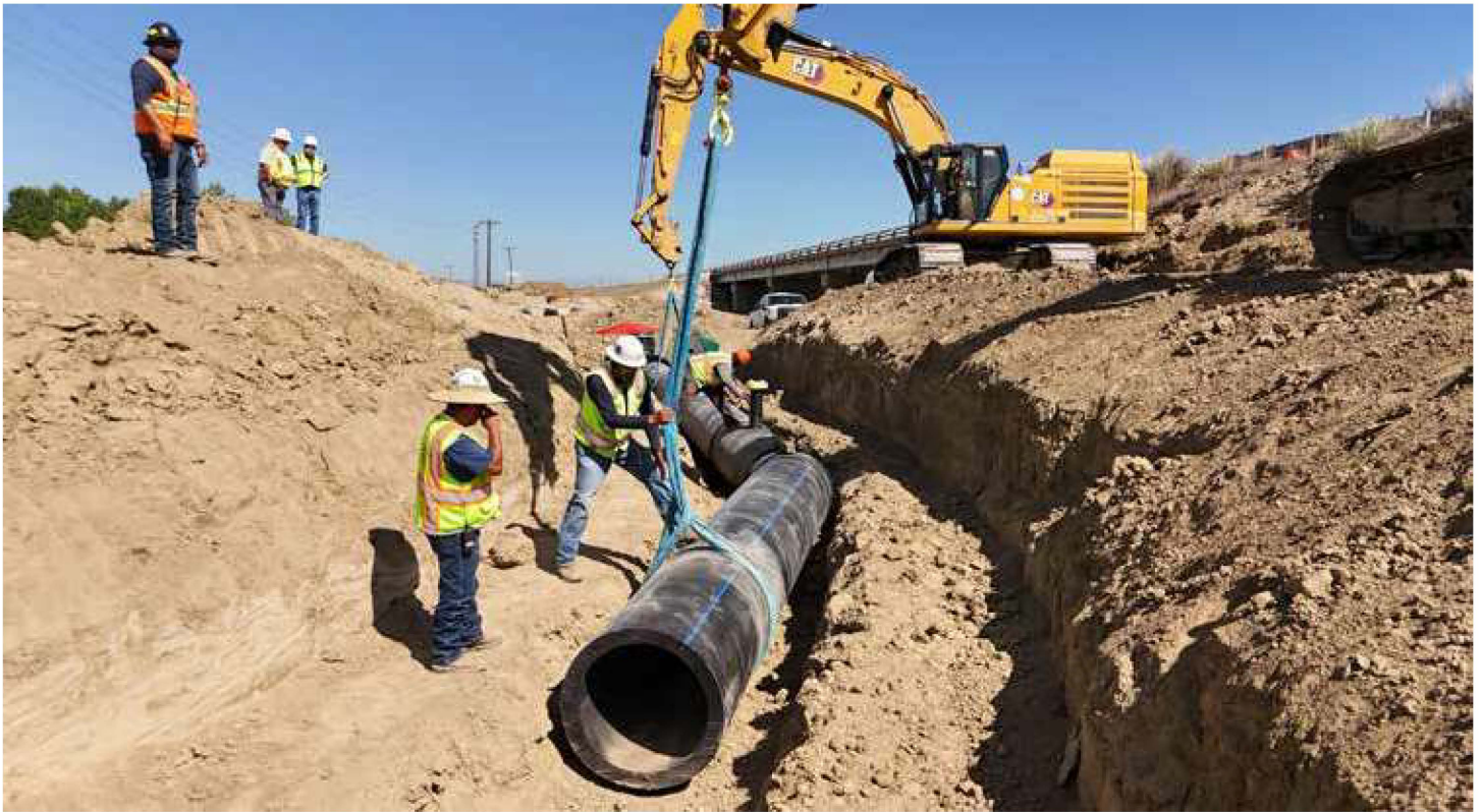
Workers from WCA Construction LLC install a section of AVC pipeline near the U.S. 50–Colorado 96 interchange near Pueblo, Colorado.
