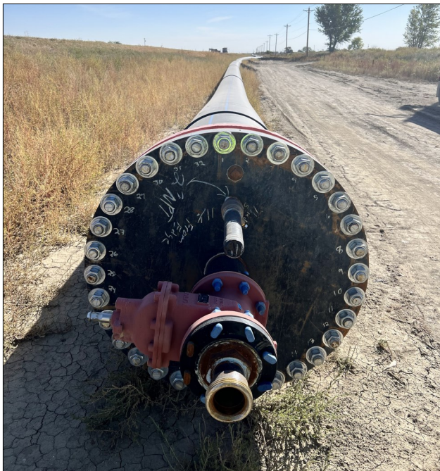
Construction continues on the Reclamation Sub-Project Boone Reach 1. A mile-long piece of 30-inch HDPE pipe weighing about 400 tons will be put on rollers and pulled through a bore hole to connect with pipe already in the ground. See more photos and details beginning on Page 4.
