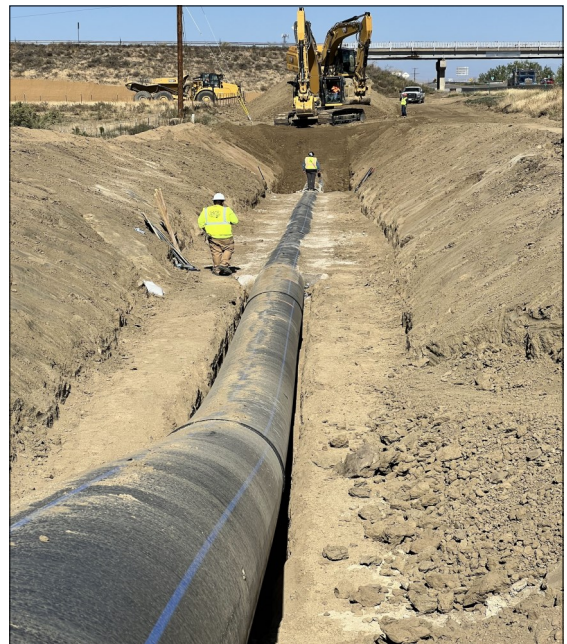
WCA Construction workers install pipe at the PuebloPlex Interchange on U.S. Highway 50.
