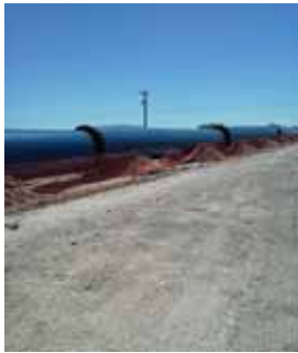
The interconnect will provide redundancy to the Southern Delivery System as well as other water connections.
