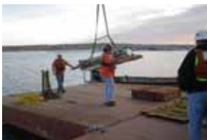
Actuator for replacement at South Outlet gate
