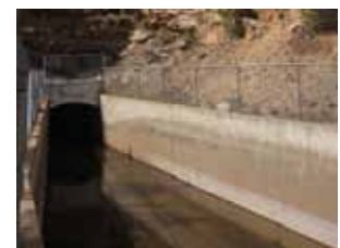
The Charles H. Boustead Tunnel conveys all the water collected in the North and South Side Collection Systems under the Continental Divide to Turquoise Lake.
