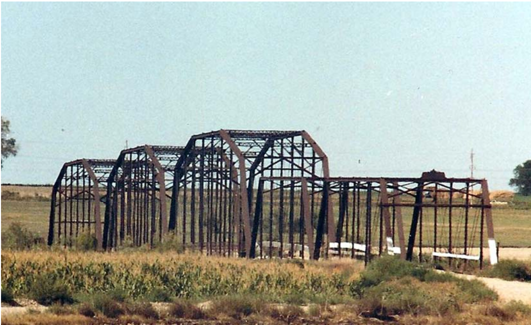
Prowers Bridge in Bent County. It is the oldest bridge over the lower Arkansas River and is Colorado's longest trussed crossing. Built in 1900 (Denverlibrary.org)
