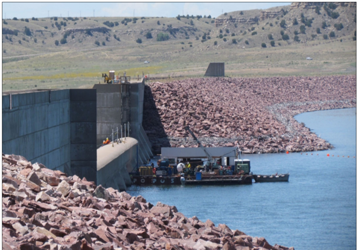
Restoration of the expansion joints between the buttresses on Pueblo Dam began in 2019. The project could cost $32 million, of which the District would pay $19 million. Reserve funds allow the District to cover its costs. (Bureau of Reclamation photo)
