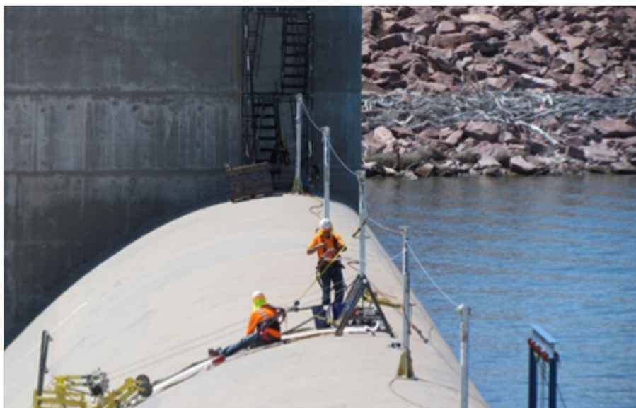
Inspection work in 2019 on the top of Pueblo Dam. (Bureau of Reclamation photo)
