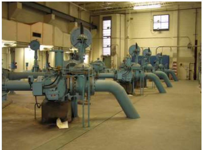
Water pumps for the Fountain Valley Conduit
