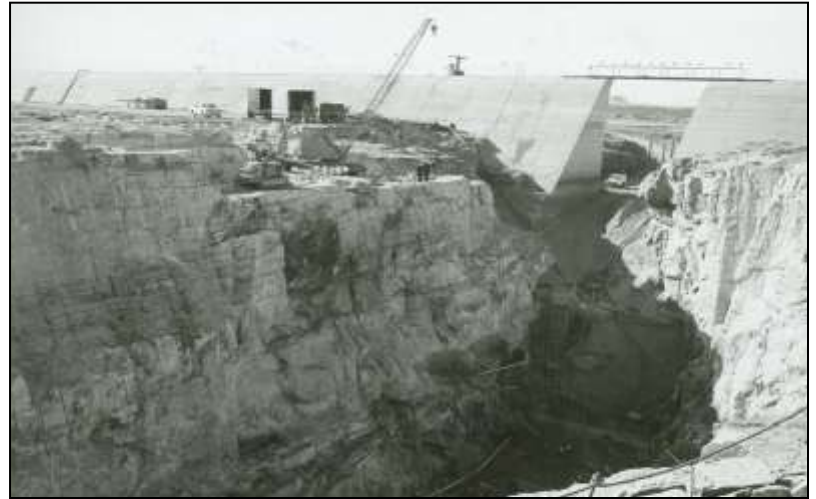
Pueblo Dam as it was being built in 1970. Shown is the buttress and spillway outlet
