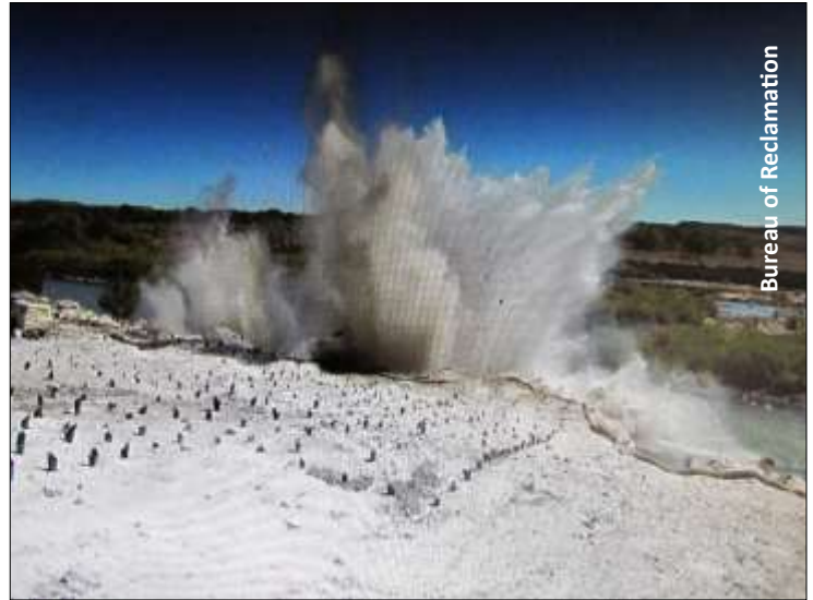
Construction begins with a blast at District hydro site near Pueblo Dam.
