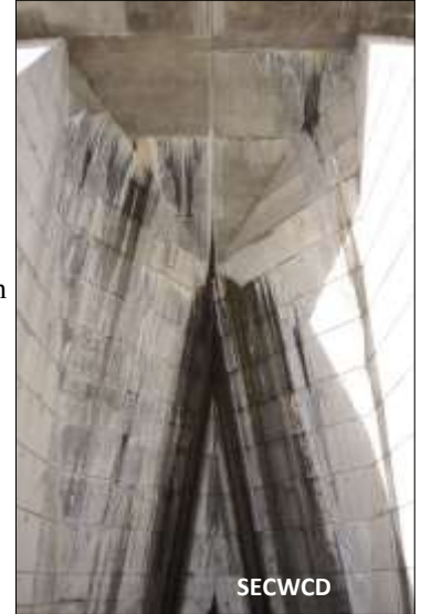
Leaking contraction joint on Pueblo Dam.
