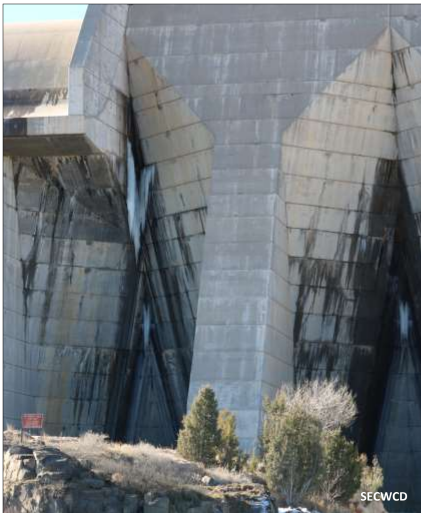
Contraction joints at Pueblo Dam are a big-ticket item for future maintenance.
